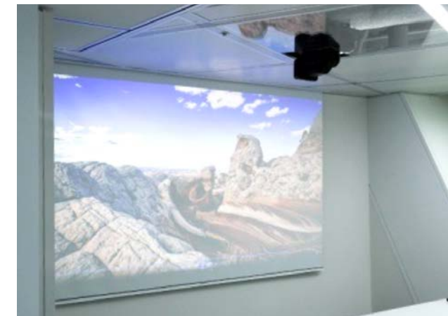
Ceiling installation EB-L1505U+ELPLX02S (1ea)
